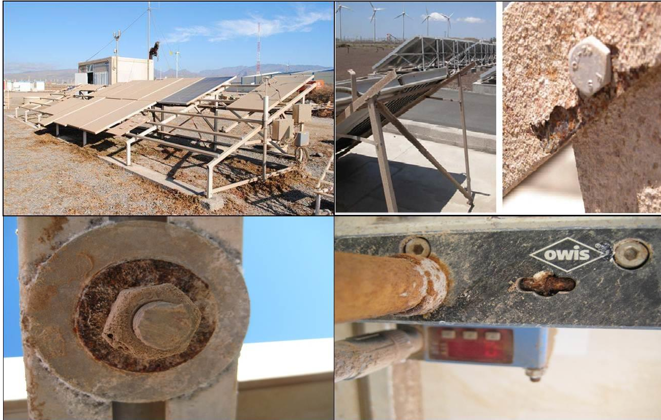
Corrosion of metal constructions
